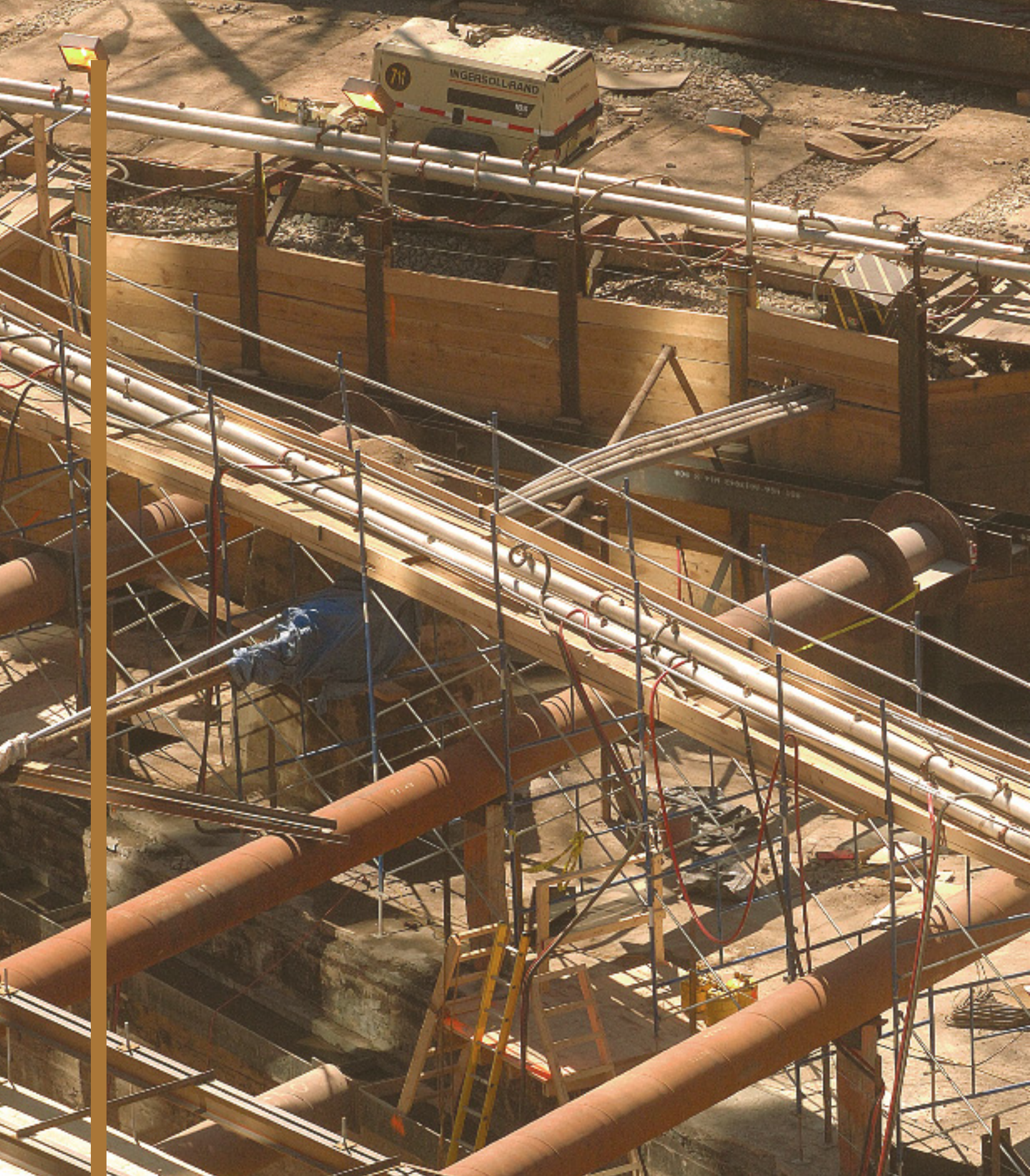
Construction of the new South Ferry subway terminal viewed from the top of the Old U.S. Custom House.
