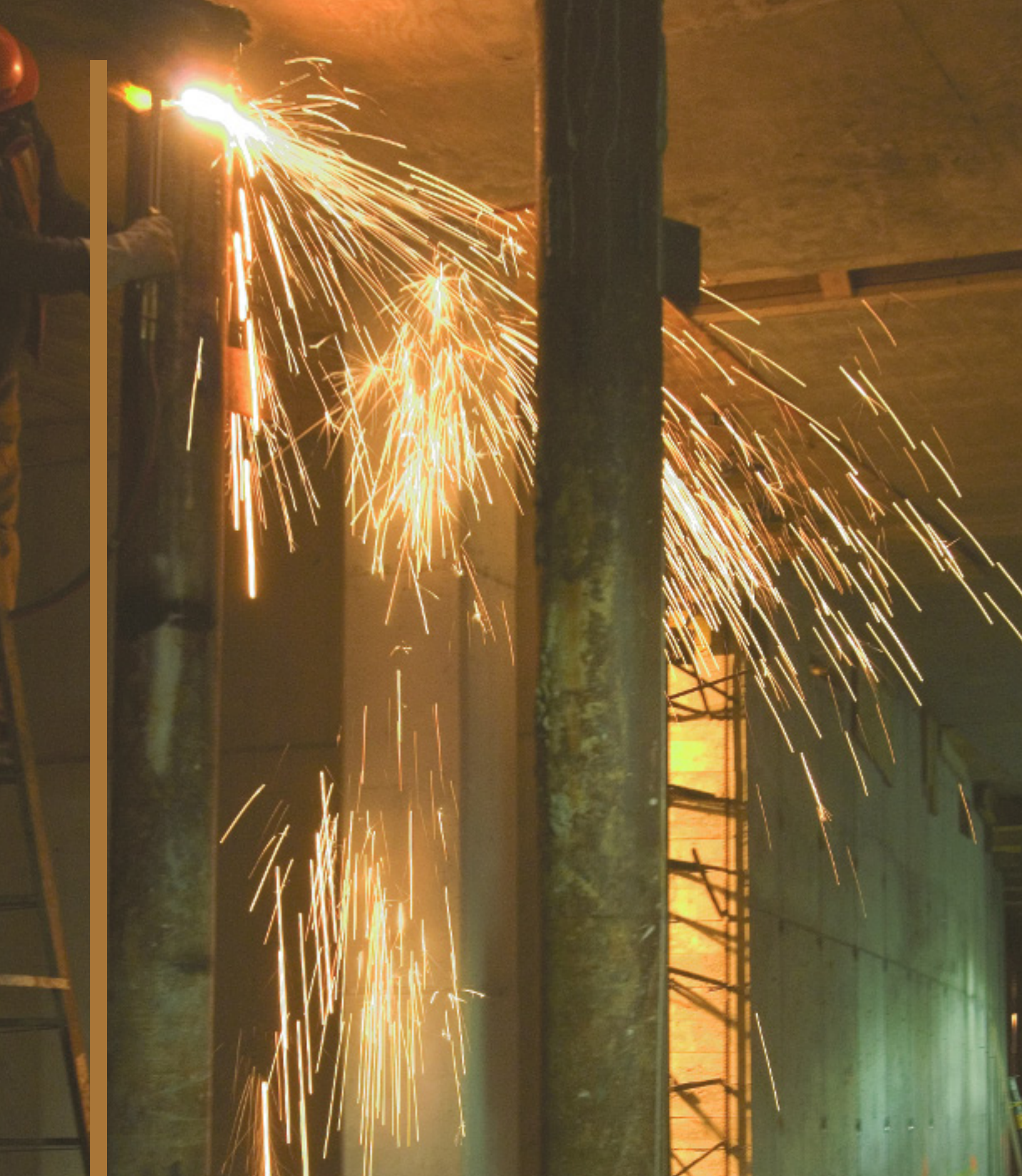
At the South Ferry terminal, a worker removes a temporary support pillar.
