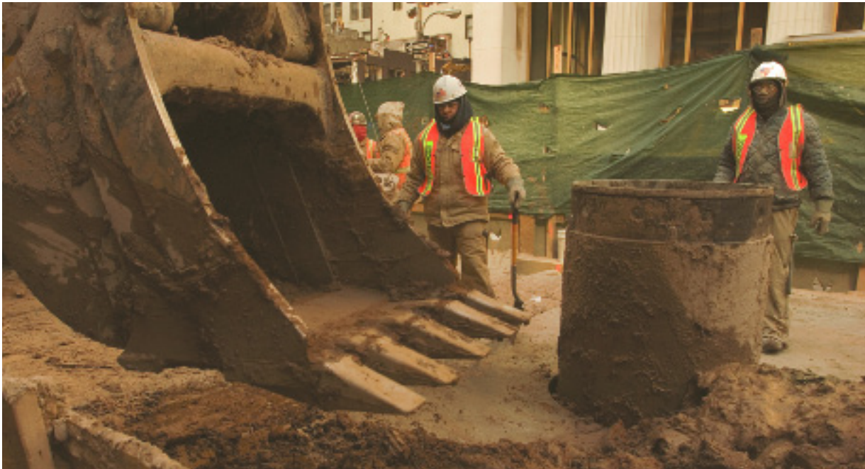
At Fulton Street/Broadway-Nassau, construction has begun on the Fulton Street Transit Center, which will improve mobility in Lower Manhattan.
