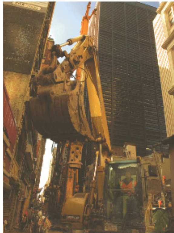
Workers have begun digging the foundation for the Fulton Street Transit Center.
