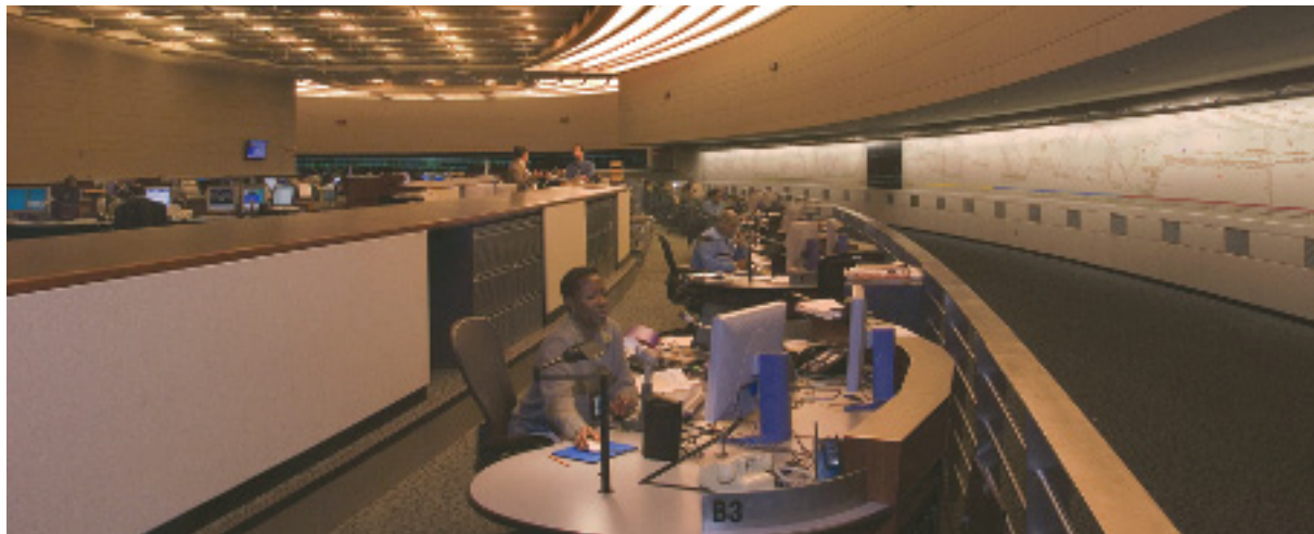
Transit's new high-tech rail control center will one day serve as the hub for all subway operations.
