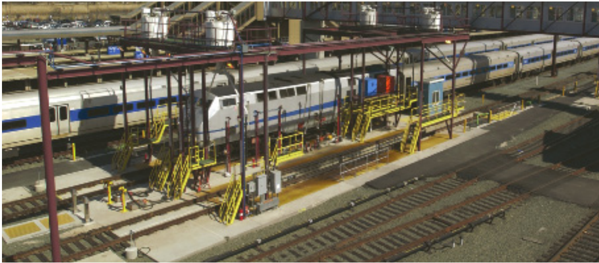
At Metro-North's Harmon Yard, a compressed air system is used to power tools and operations. When fully operational, it will save 350 kilowatts annually.
