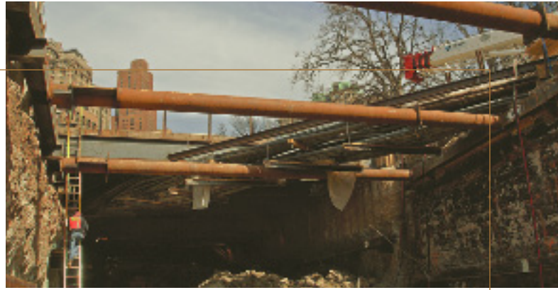
When completed in 2008, the new station at South Ferry will provide a two-track terminal for the 1 line, improving service in Lower Manhattan.
