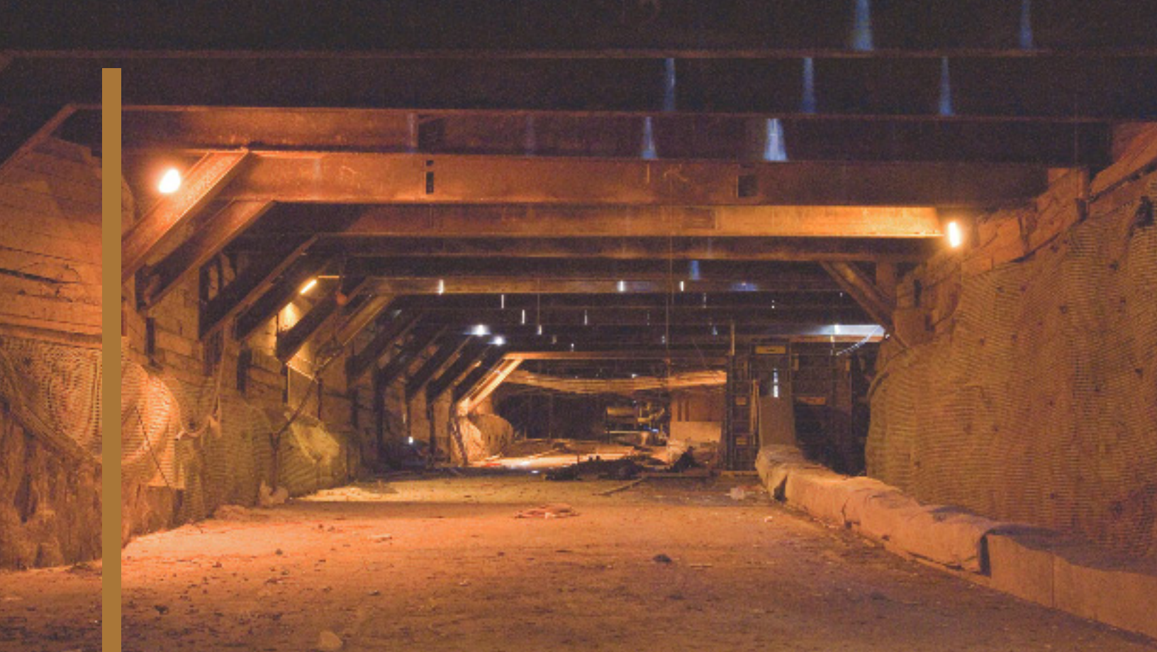
Tunnel work is progressing at the South Ferry station. The new 1 line terminal will open in 2008.
