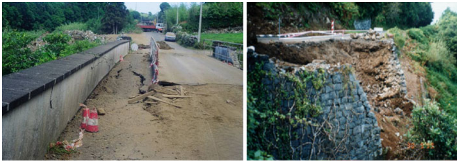
Fig. 6 Damage to pavement and retaining wall
