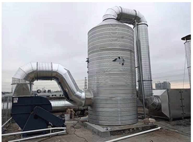
Brother Technology (Shenzhen) Ltd.: VOC treatment system
