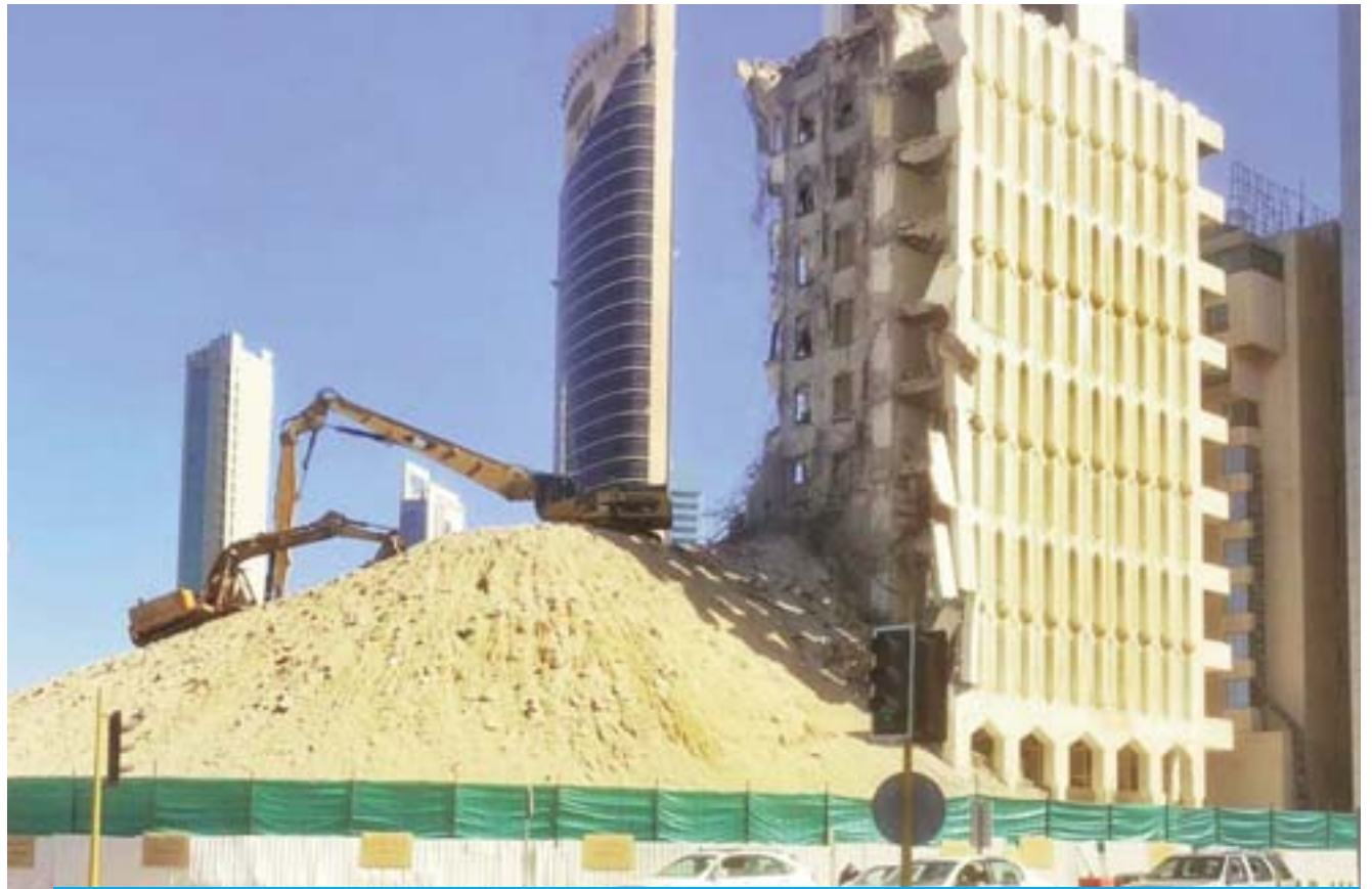
The demolition of the old Kuwait Airways building has resumed in Kuwait City. Demolition was halted after a June 2015 accident where an excavator fell several floors, killing the operator. — Photo by Kuwait Times
