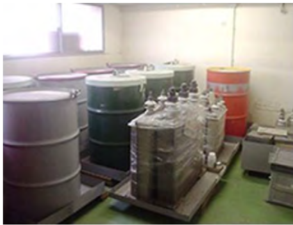
Inside the polychlorinated biphenyl storage warehouse at the Headquarters in Kawasaki
