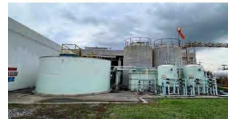
Chemical wastewater processing facilities (FGT)
