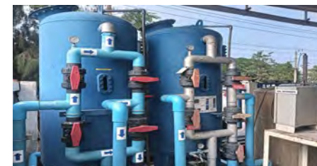
Oil skimmer and carbon filter tank used in wastewater processing systems (TCFG)
