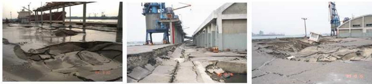
Fig. 2 Results of liquefaction of backfill behind quay wall following Chi-Chi earthquake
