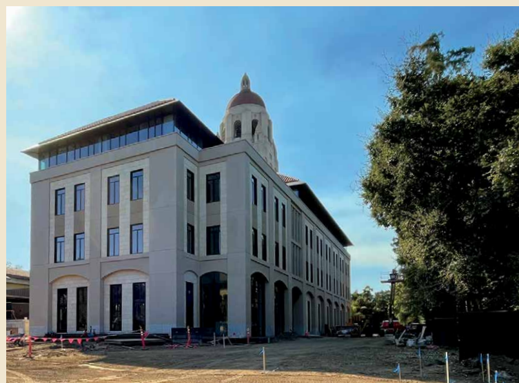
View of the the George P. Shultz Building, to be dedicated in February 2024, under construction PHOTO: HOOVER INSTITUTION, 2023
