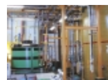
Wastewater treatment facilities
