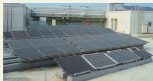
The PV power system on the roof of the new TET premises
