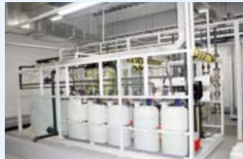
RO*1 water treatment room
