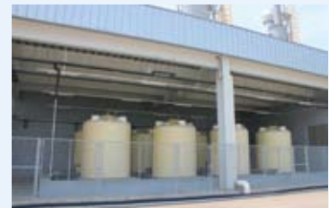
Liquid chemicals storage tanks
