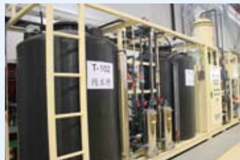
Pure water production equipment
