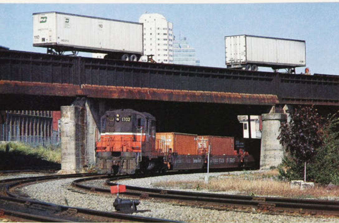
As Conrail train TV-6 thunders by overhead, P&W 1702, its only GP9, returns from CR's East Worcester Yard with container cars.
